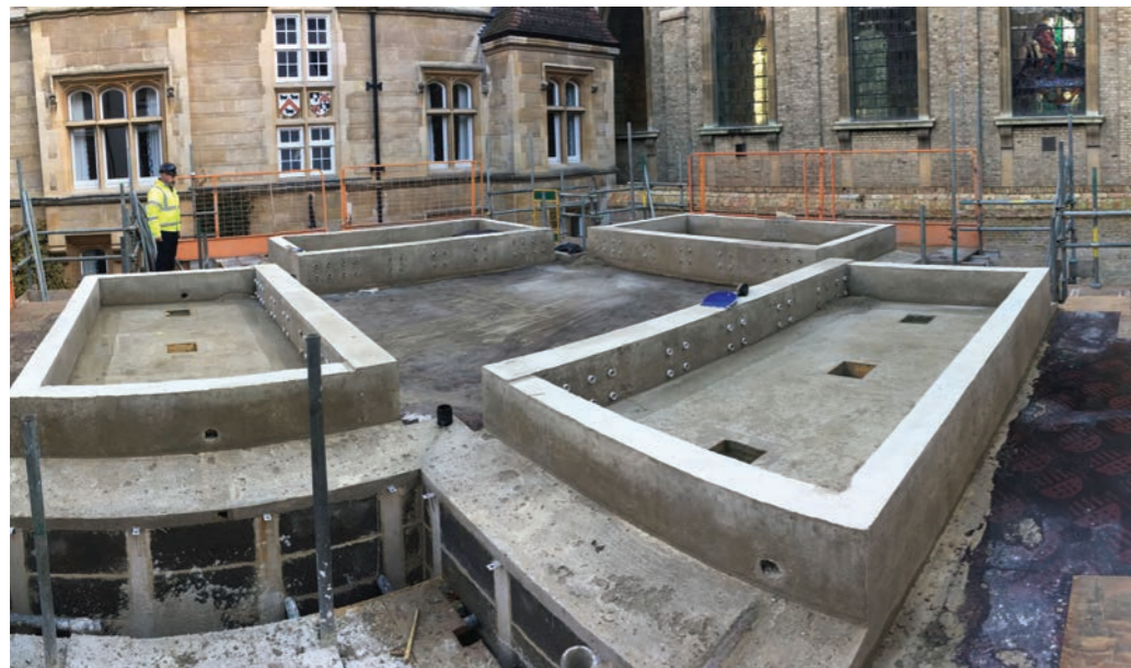
Left: Severely restricted access to the 17x22 metre site meant that the only piece of powered machinery available was a mini digger. The rest of the work relied on manual labour.
